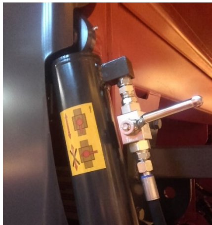
Picture 282. Lifting cylinder safety valve closed.
